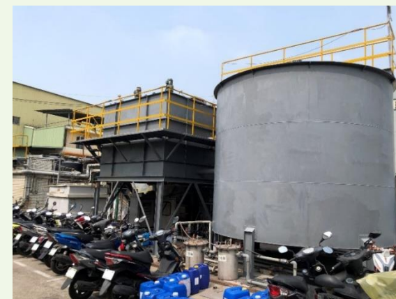
Taiwan Headquarters Wastewater Treatment Facilities
