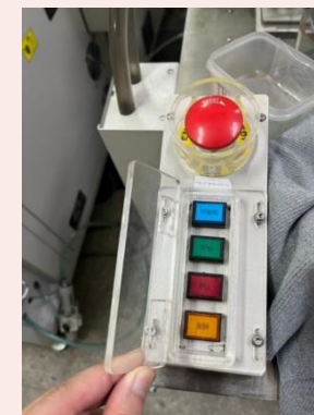
Improvement of operation switch area
