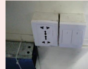
Improvement of sockets
